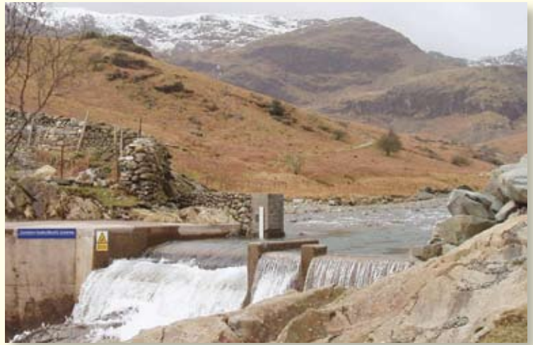
A micro-hydro installation above Coniston in the Lake District
