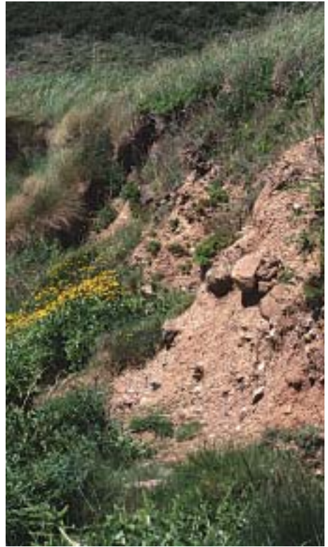
Slowly-eroding 'head' cliff, Overton. Mike Edwards
