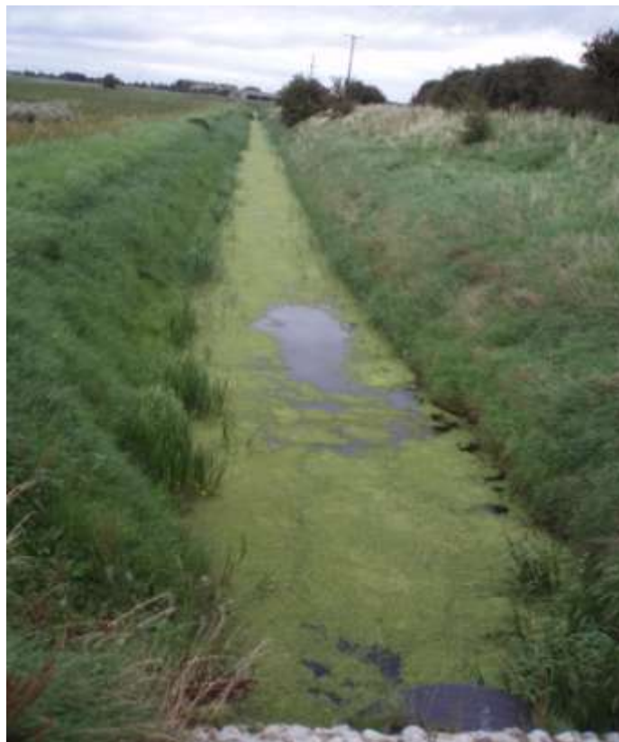
Plate 8 The Old Sea Drain taken from the Pinchbeck Marsh Pumping Station
