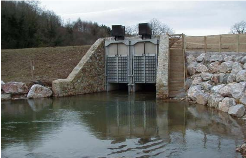
Figure A4.20. Sluice gates on the down stream side of the dam. In the foreground is a specially created pool for fish. Note how the dam structure has been naturalised as much as possible, and incorporates nesting facilities for dipper.
