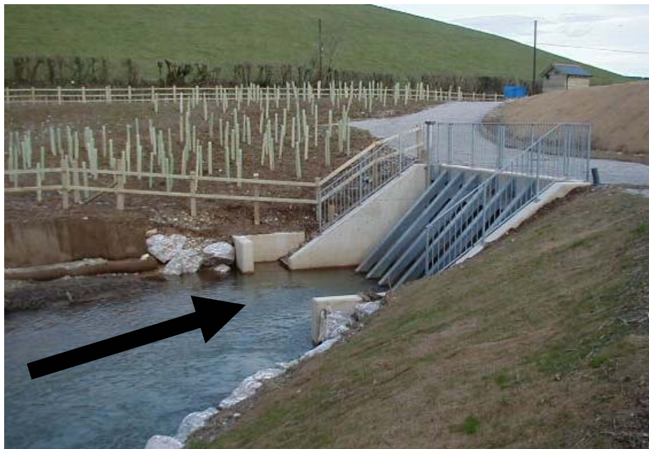
Figure A4.21. Upstream side of the dam includes the culvert structure. Note the newly planted broad leaf trees in the background.
