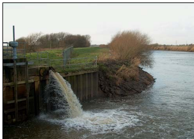
Figure 2.8 Beckingham Pumping Station
