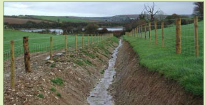
New fencing controlling access to creek. Shellfish beds are in the creek which can be seen directly at the end of the watercourse
