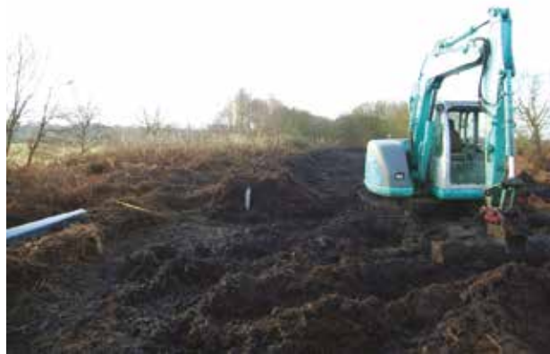
Figure 1. Installation of plastic piles as part of bund creation on land adjacent to Astley Moss. The works created a new “lagg” fen to reduce the hydrological gradient off the moss so helping re-wet the core of the bog.
