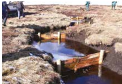
Figure 15. Wooden dams installed by NT volunteers in gully on blanket bog. South Pennines. Some were lost subsequently in moorland fires, others began to erode underneath and round the sides, whilst the best still hold water. It is not always easy to install effective dams. (Photo: Penny Anderson)
