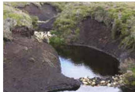
Figure 16. Stone dams in deep gully, raising water table in a number of stages. Peak District. It will take many years before the water table is close to the surface in such situations. (Photo: Penny Anderson)
