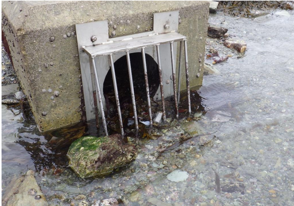
Figure 17. Land drain at Looe
