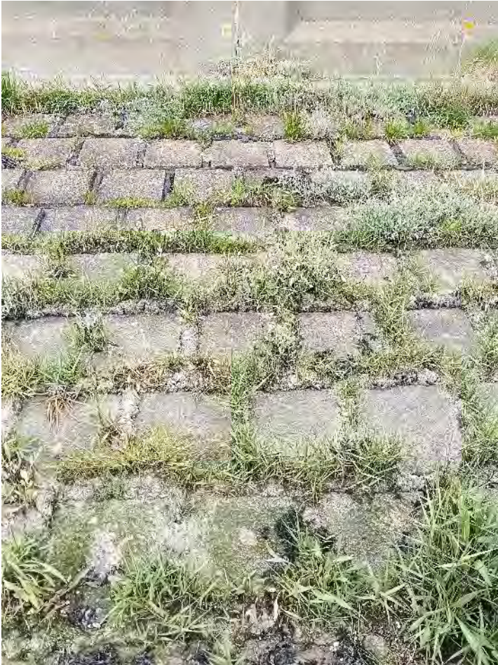
Plate F1.11. Older-style block facing on the seawall in the central part of F1 with Atriplex portulacoides , Plantago maritima and Spartina anglica in the joints.
