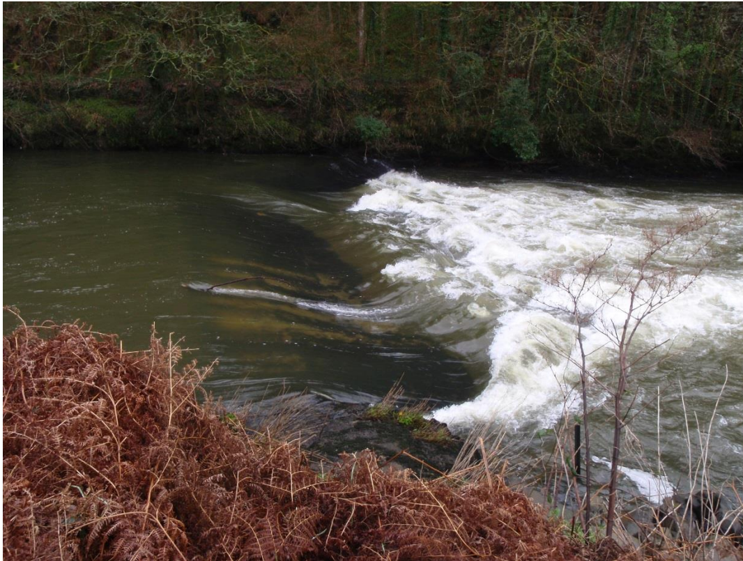
Figure 11. The weir at the head of Cottage Run is a migratory barrier to smelt except at high water on spring tides.
