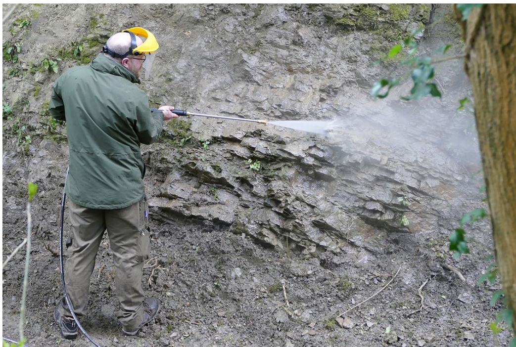
High pressure wash – Wagon-way, January 2018. High pressure water lance being used to remove soil and recalcitrant vegetation from exposures. ©Dudley Metropolitan Borough/ Graham Worton reproduced with permission
