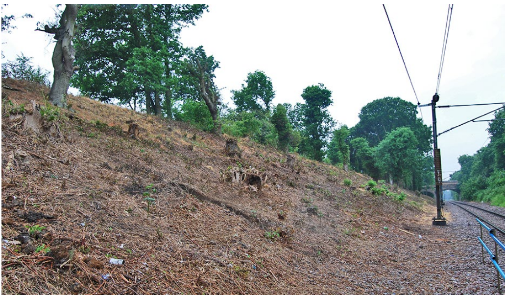
A view along the railway cutting at Hornchurch after the vegetation clearance had taken place. ©Natural England/Emily Dresner
