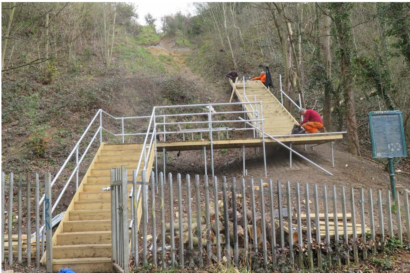
Gilbert's Pit - step construction in progress in area of scree build-up and slide. ©Laurie Baker reproduced with permission
