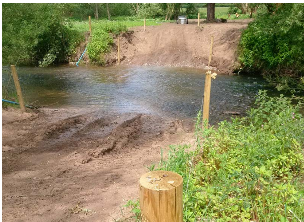
Damage to river bank and flood plain of inner side of meander caused by excavation for a track to connect adjacent grazing areas. ©Natural England/Anna Wetherell
