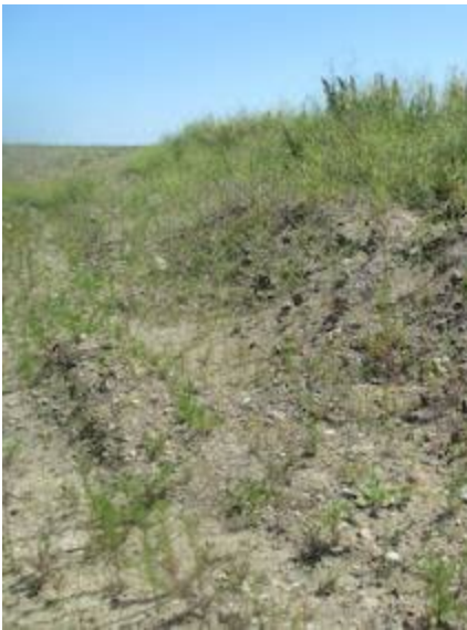
Photo 34 - partially vegetated spoil compartment D
