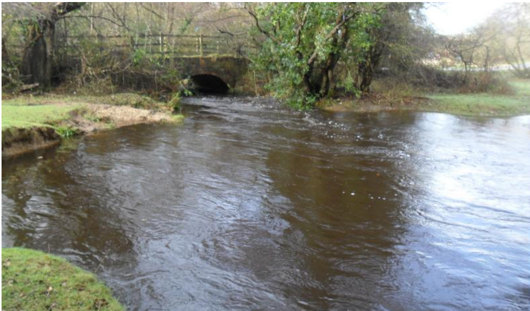
Figure 1-7: Flow concentration and hydromorphic alteration at Wooton Bridge.
