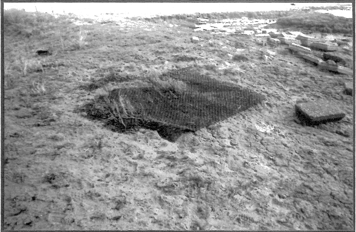
Photograph 15: February 1995 Erosion of sea wall adjacent to the spillway exposing geotextile fabric
