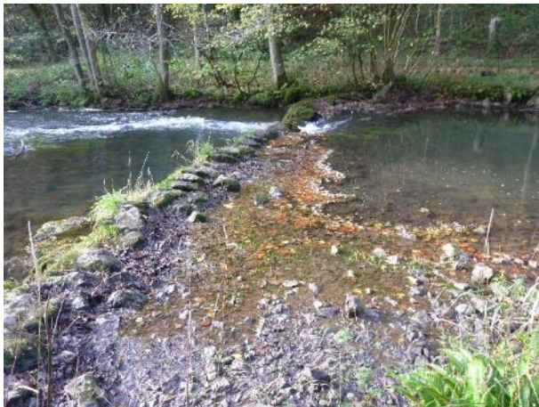
Weir has been breached naturally. Remove introduced stone.
