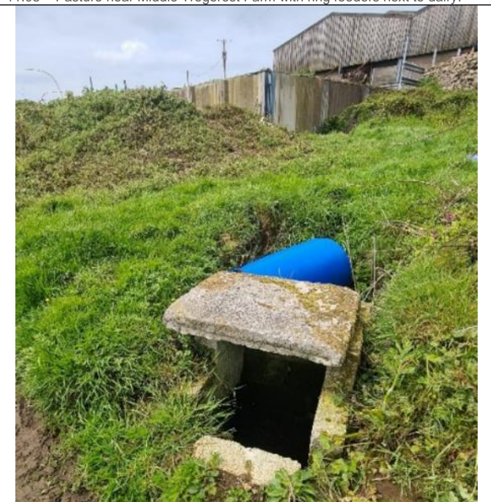
11.07 – Drain at bottom of slurry tank (slurry tank in background) with brown water dripping into an underground pipe.
