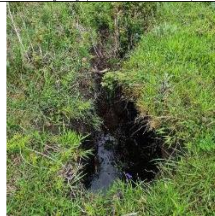
4.11 – Chamber of collapsed large peat pipe carrying water along flow pathway.
