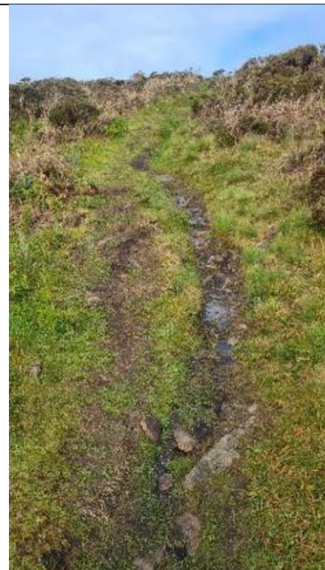
5.06 – Flow seepage on steep footpath.
