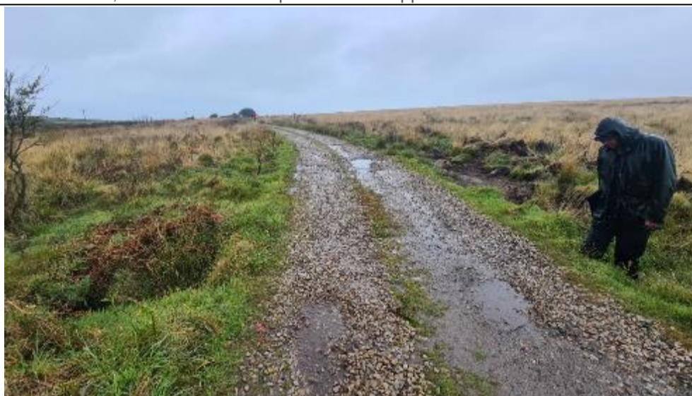
1.05 – Flow pathway leading from semi-natural rough ground on the right of the image, through the culvert under the track, to the mire on the left of the image.
