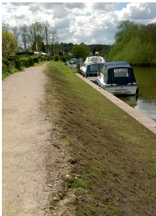
Examples of erosion and revetment works on the Thames Path at Hurley
