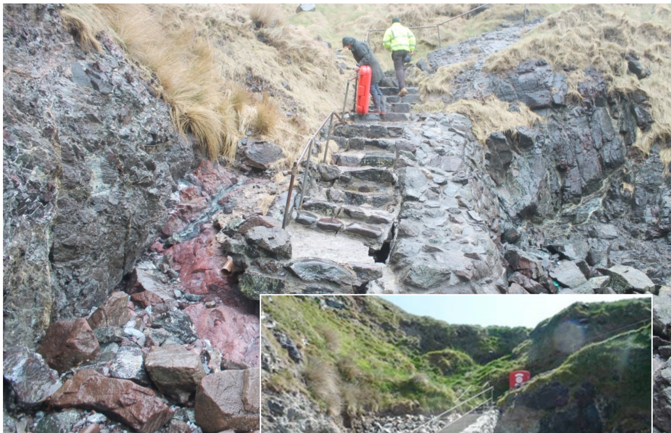
BEFORE and AFTER: Step repairs on the South West Coast Path at Kynance
