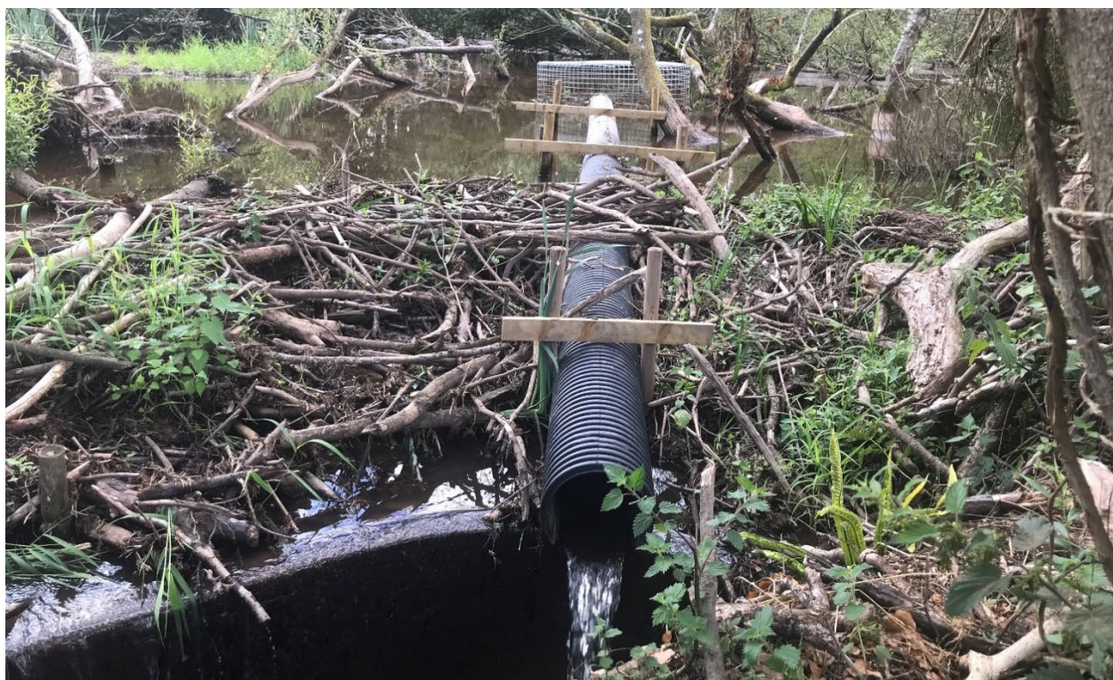
Figure 6: Flow device with a cage at the inlet installed through a beaver dam to manage water levels. Credit: Giles Wagstaff.
