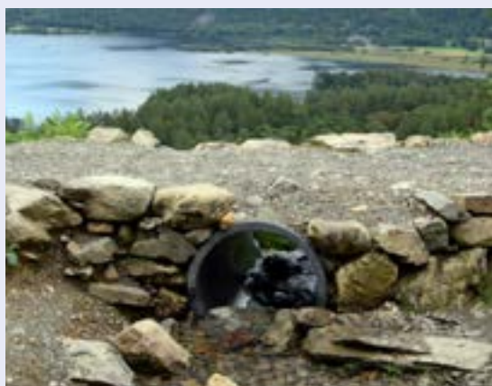
Repaired section of Cat Bells path with improved drainage culvert. © Natural England/A Mackintosh
