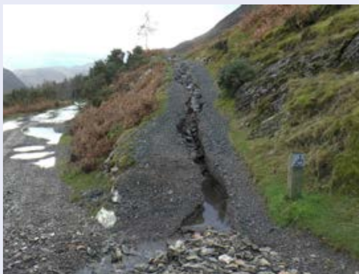
Storm damage on Cat Bells footpath. © Jessie Binns, National Trust
