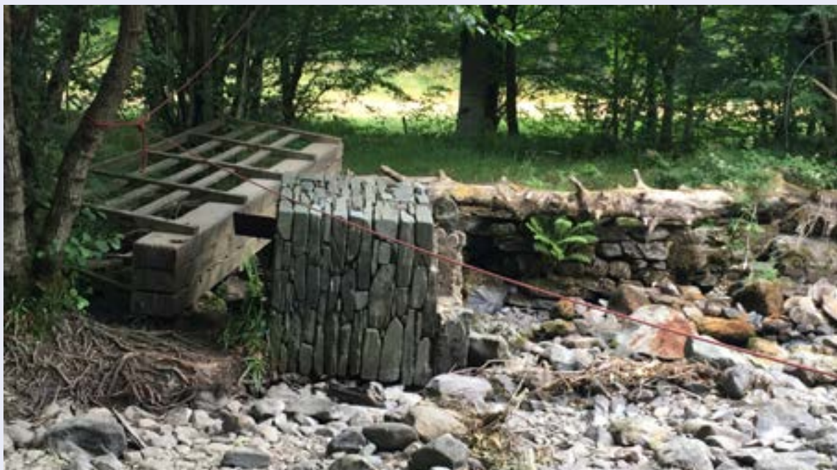
Damaged bridleway ford and footbridge at Townend © Natural England/A Mackintosh
