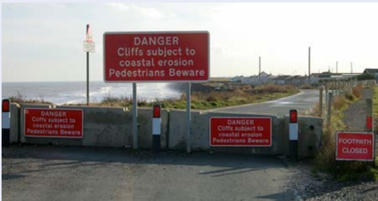
Coastal erosion to roads and footpaths in the East Riding of Yorkshire. © Natural England/A Mackintosh
