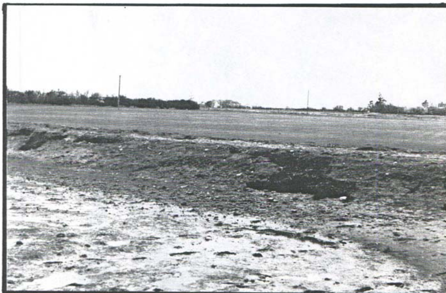
Plate 3. View of eastern wall erosion, geo-fabric exposed at several locations (see Plate 4).
