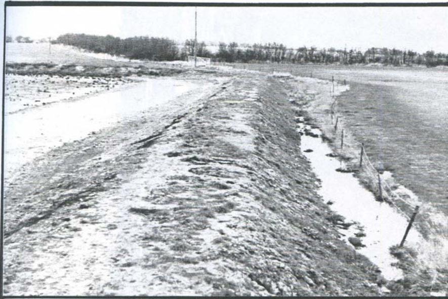
Plate 2. Enclosure wall at east end of site. Note severe erosion on western face and increased level of seepage at foot of wall
