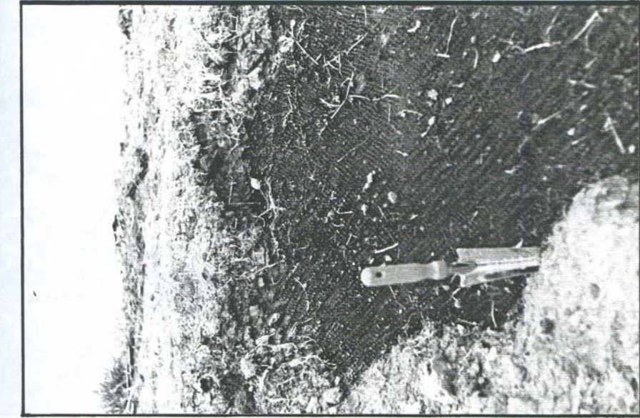
Plate 4. Close up view of extensive erosion and exposed geo-fabric
