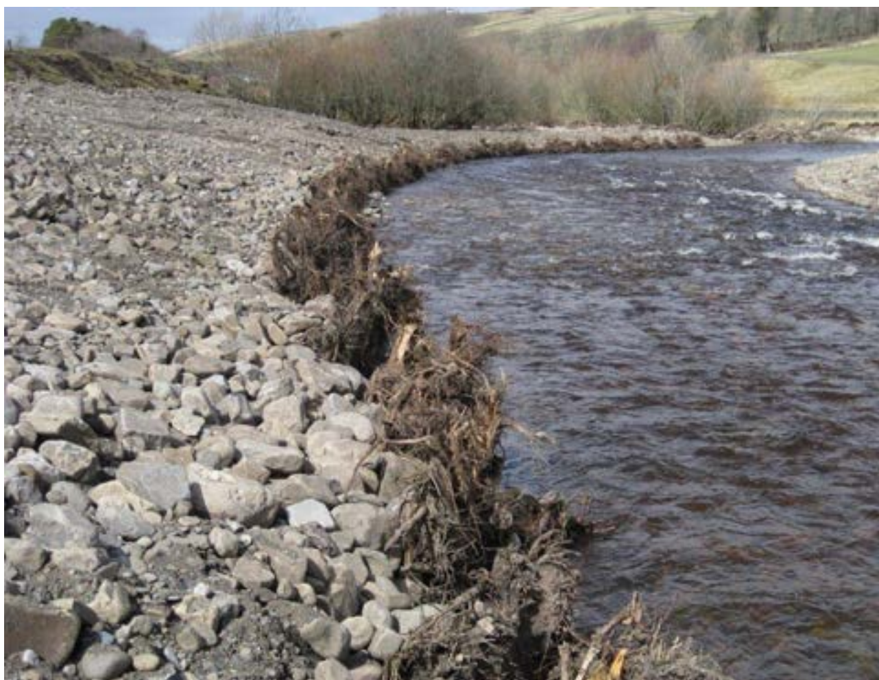
Engineered 'log jam' - soft engineering solution preventing erosion of the nationally important Tynebottom Mine spoil (River Tyne and Tynebottom Mine SSSI). © Natural England /Simon Stainer
