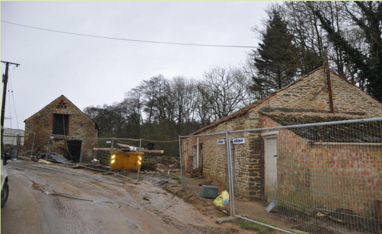
Coulton Mill HLS Heritage Restoration project inundated with sediment from Coulton Bank
