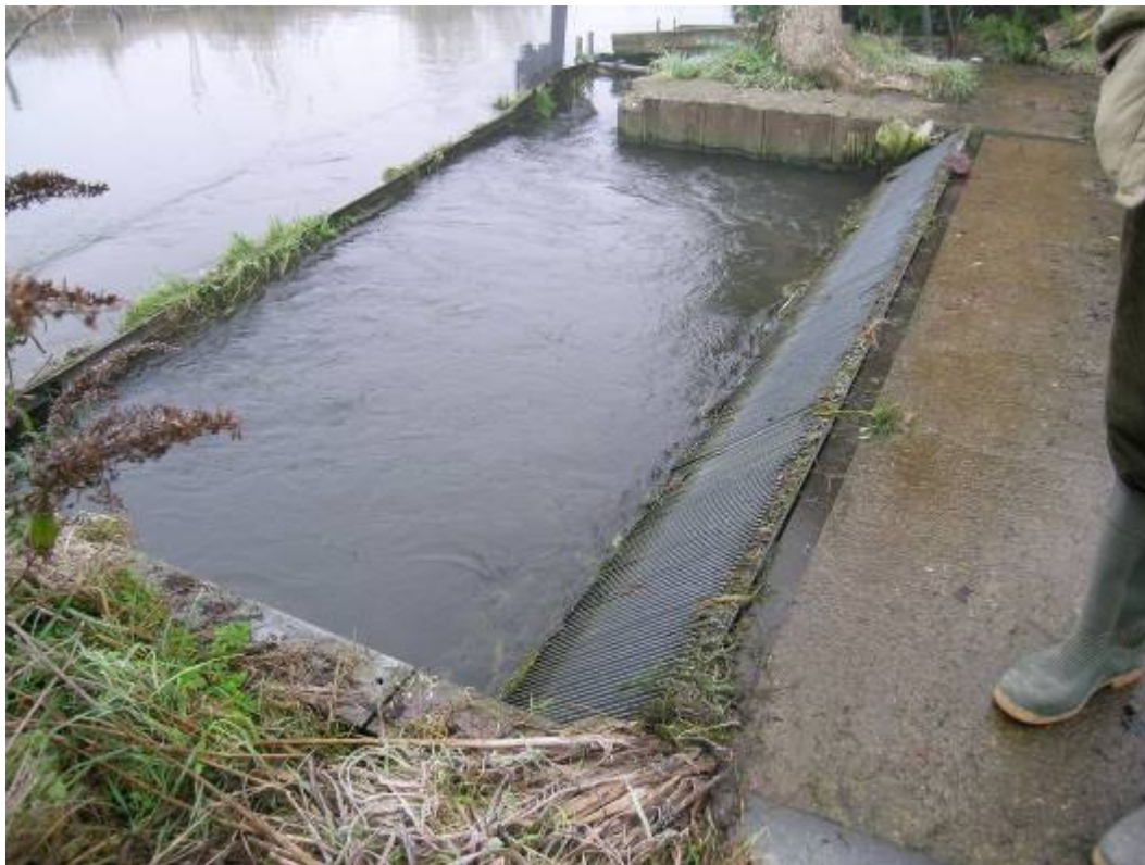
Figure 7.2. A bar screen on the intake for a trout farm on the Avon. The gap between the bars, around 10 mm, is sufficient to exclude salmon smolts. Although the screen material itself is fairly cheap there are major engineering costs associated with effective and safe installation on intakes handling sizeable flows, and maintenance is required at least daily to keep the screen clear of debris.
