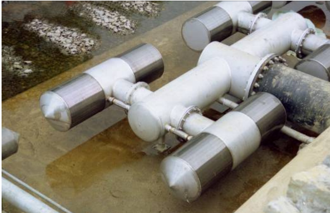
Figure 7.1 A Johnson Passive Wedge Wire Cylinder (PWWC) Screen on a water intake on the River Tamar, dewatered. This is one of the few practical screen types for utilising fine mesh and small gaps. The slot size in this case is 3mm, which would exclude cyprinids of 50 mm and larger. The screens are kept clear of debris by bursts of compressed air released inside the screen cylinder, triggered automatically by a pressure drop across the screen. The costs of supply, installation and operation make the deployment of such screens quite impractical in the situation being considered in this report.
