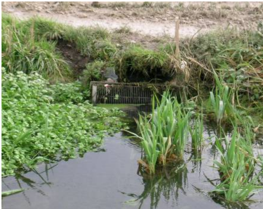
Figure 7.3. A simple bar screen on an intake to a single pond on a trout farm on the Avon. In contrast to the situation shown in Figure 7.2 installation costs for intakes handling such a limited flow can be modest. Regular maintenance is required to clear the screen of debris, but this is less of an issue if the effectiveness of the wetland being supplied is not dependent on a constant flow.
