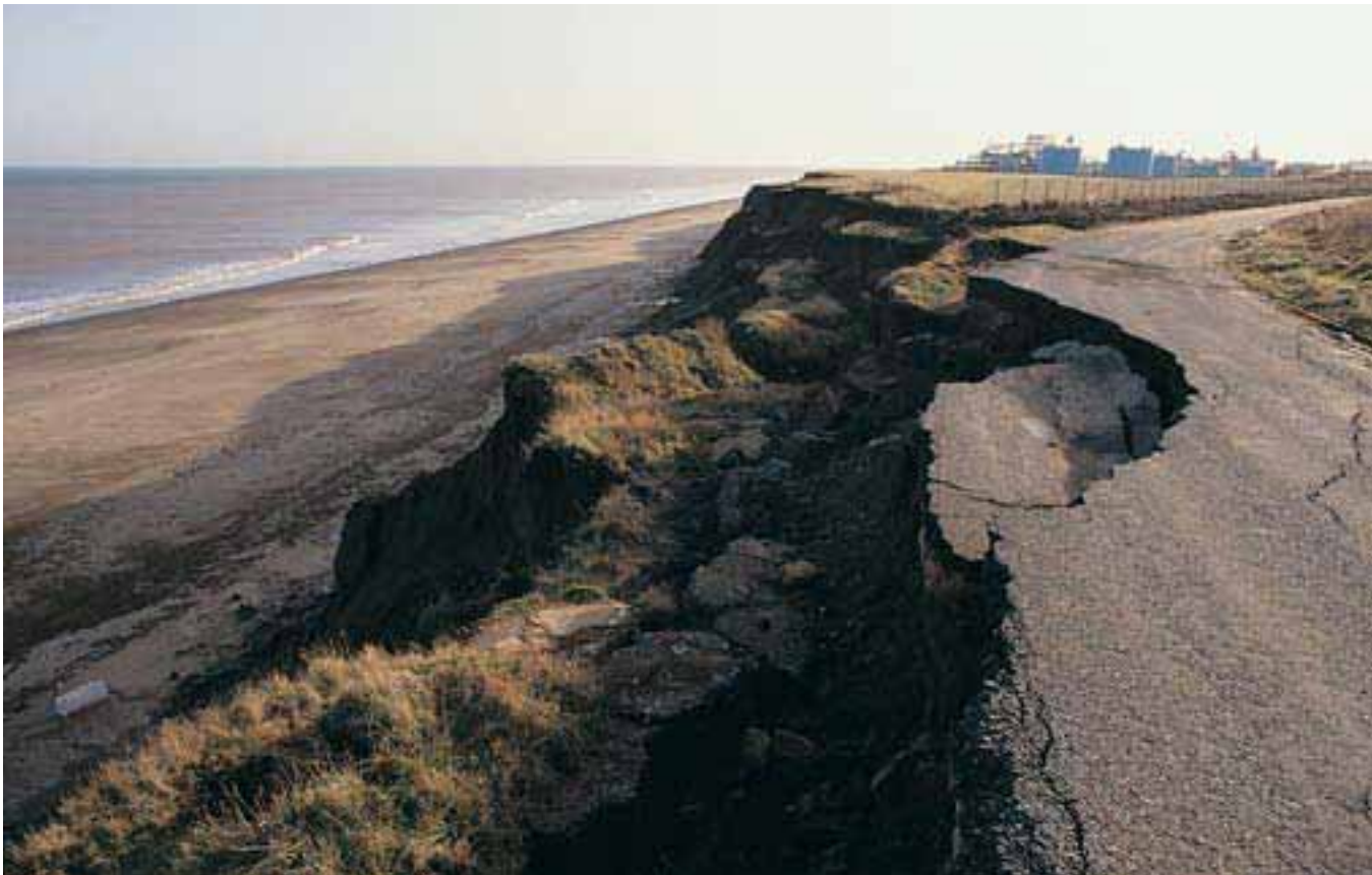
Coastal erosion threatens this gas terminal on the Holderness coast.
